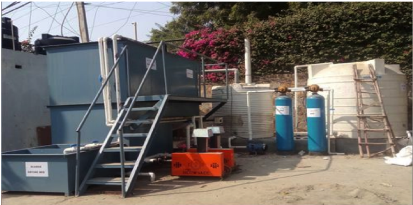
Figure 35: Fluidised Aerated Bed
