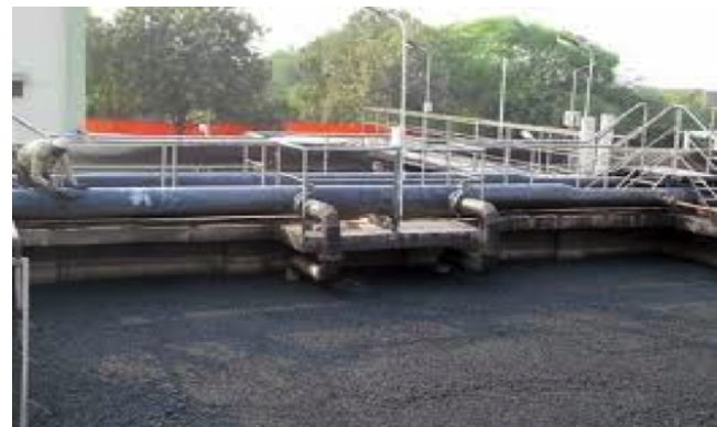
Figure 36: Photograph of a Moving Bed Bio Reactor plant
