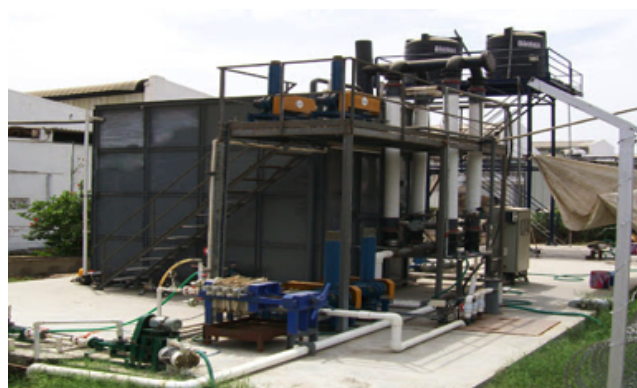
Figure 38: Photograph of Membrane Bio-Reactor Plant
